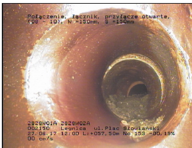
Foto 153 Video: CD1 Stan BCA A A 57,50 m 8 - 10 o'clock
